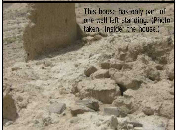
This 2-room house was hit by flash flood water racing behind it. (Photo taken from the back of the house.)
